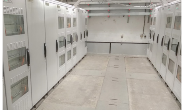
Engineered Safety Feature Actuation System at South-Ukraine
